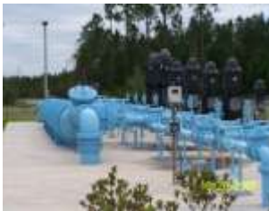
High Service Pumps
