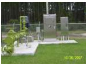
Raw Water Well Pump
